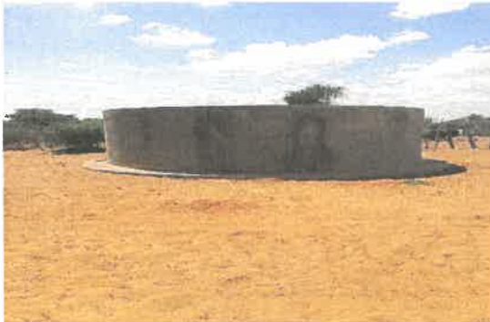
Reservoir to be repaired at Magonate -JTG
